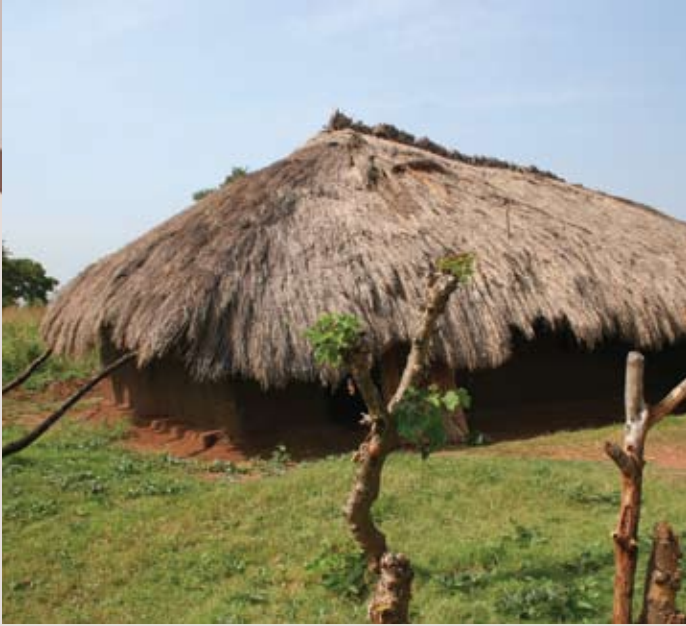
Dilapidated ATC classroom
